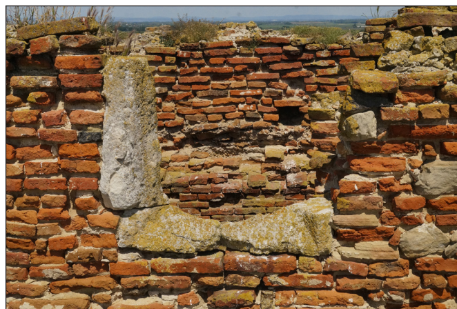
Fig. 10. South-eastern window on the third floor before restoration
