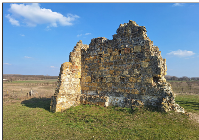
Fig. 9. The north wall prior to restoration – cracks running through the wall, spalling on the plinth, crumbling wall crown, and heterogeneous pillar infill dating from 1999 (photo: Bálint Kelemen)
