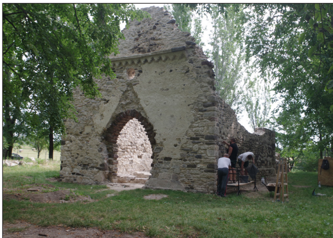
Fig. 4. The ruin church from the southwest during the ruin conservation works in July 2023
