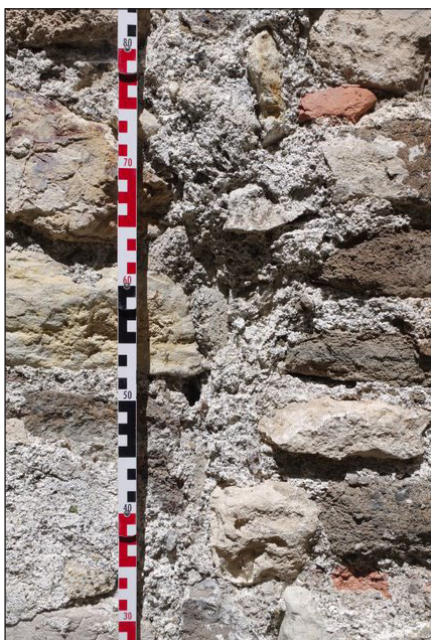
Fig. 6. The joint in the north wall of the nave with parts of an oblique surface in May 2022
