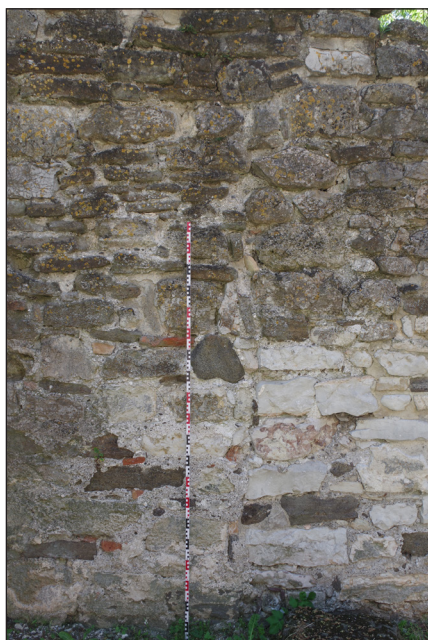
Fig. 7. Vertical wall joint in the eastern section of the south nave wall
