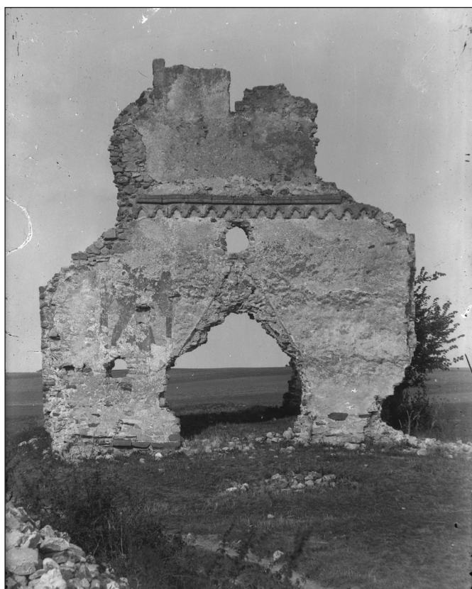
Fig. 9. The western façade on a photo from the late 19th or early 20th century with fresco remains on the northern side of the western nave wall and the stub of the tower in the upper part of the façade (Historical Monuments Photo Collection 033.500aN, GEREVICH 1938, 57. t.)
