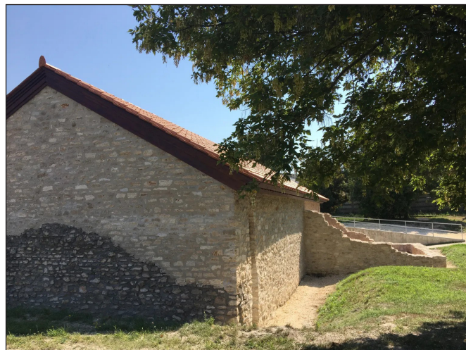
Fig. 8. The protective building of the Symphorus Mithraeum in Aquincum (Óbuda, Budapest, Hungary) (photo by the author)
