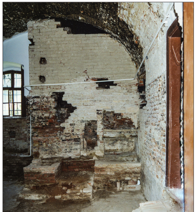
Fig. 1. The excavated kitchen of the Deák House in Söjtör (research by András Koppány, 2002)
