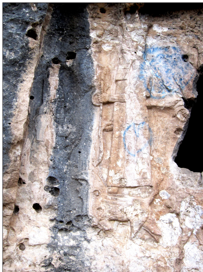
Fig. 3. Detail of the Assyrian relief; the damage by weathering and graffiti is clearly visible
