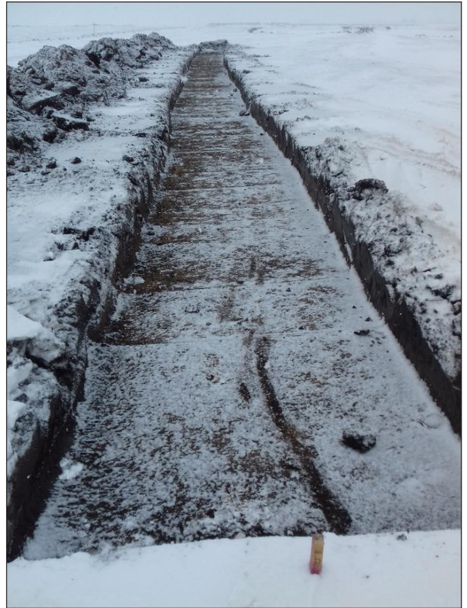
Fig. 1. Excavations realized in the frames of PADs are not always carried out in ideal conditions
