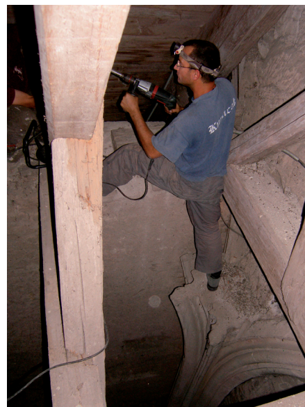
Fig. 2: Drilling of a core sample from the roof structure of the Lutheran church in Sebeș
