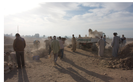
Fig. 1: Excavation of the debris covering the forecourt of TT -400- (photo by Balázs Tihanyi)
